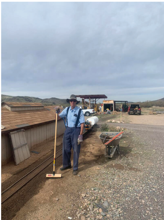
Bill Mellors is busy getting ballast on new track into the MoW container.
