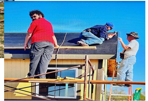
Tim, Bob and Perry work on the roof. Gary also. Taking photos!
