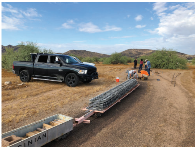
Dakota, Tim and Perry help bring the straight sections of track out to be connected together. Thanks Dan, for the photos.
