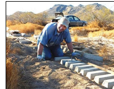
Tom Harrington, seen here learning how to lay cement ties, is the newest member on the Board of Directors.
