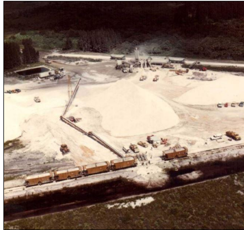
Construction of the Space Shuttle runway. Source: Historical Survey of KSC Railroad, Archaeological Consultants, Inc.
