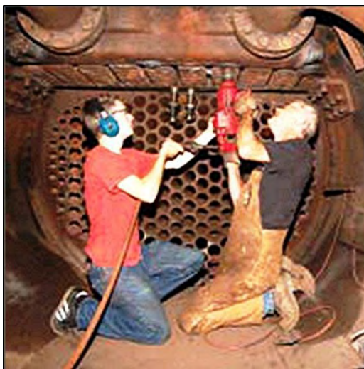
(left) Restorers work on a superheater header. The viewer is looking from the front of the smokebox toward the front flue sheet. Photo: Bruce Miller, Cooper Mountain Photography
