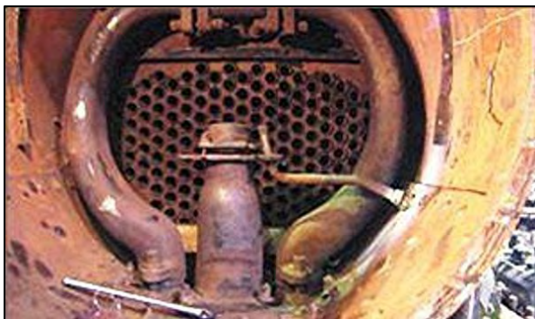
(above) The front end of a smaller locomotive where there is no superheater header.
