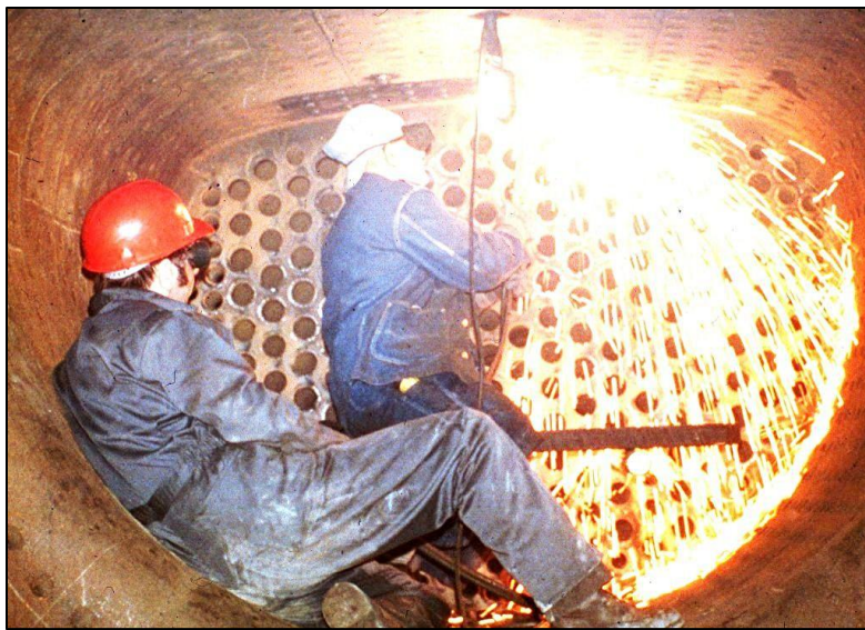
A worker welding on the SP 4449's boiler tubes during the rebuild in 1975 for the American Freedom train.
