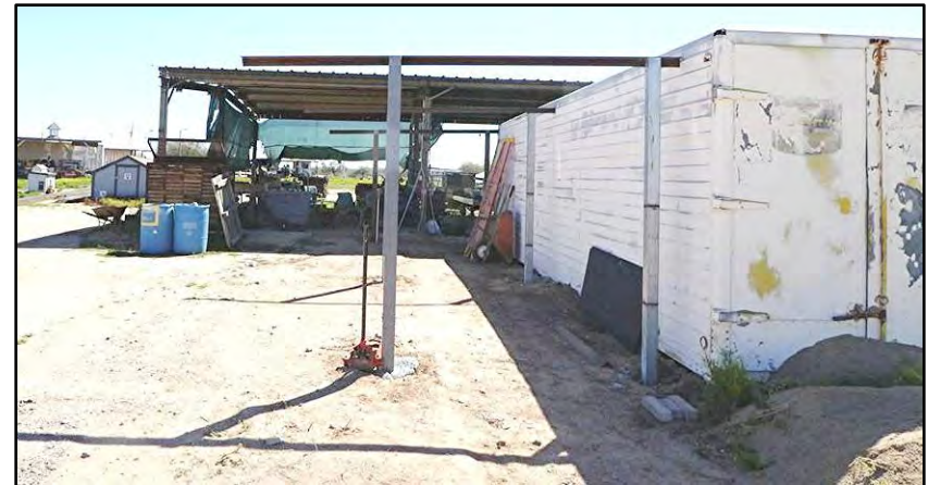
The Sawmill Container (north side) where the supports have been installed for a cover to protect the golf cart parking /charging area.
