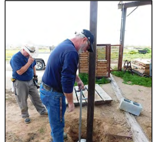
Pete Pennarts and Matthew Rockwell setting a post for the shed to store golf carts.
