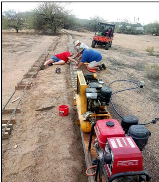
Finishing the last of the concrete ties on the Pottsville Branchline – Joe Schnyder, Cliff Fought, Matt Rockwell and Dave Kulman – just in time for the Fall Meet.
