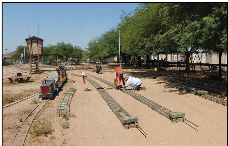
These new spurs include red posts with outlets for charging electric trains. Daniel and Scott were there along the way to help out with Joe. This took many hours of hard work in the Arizona heat. Thanks to these hard workers, it will be less congested during meets.
