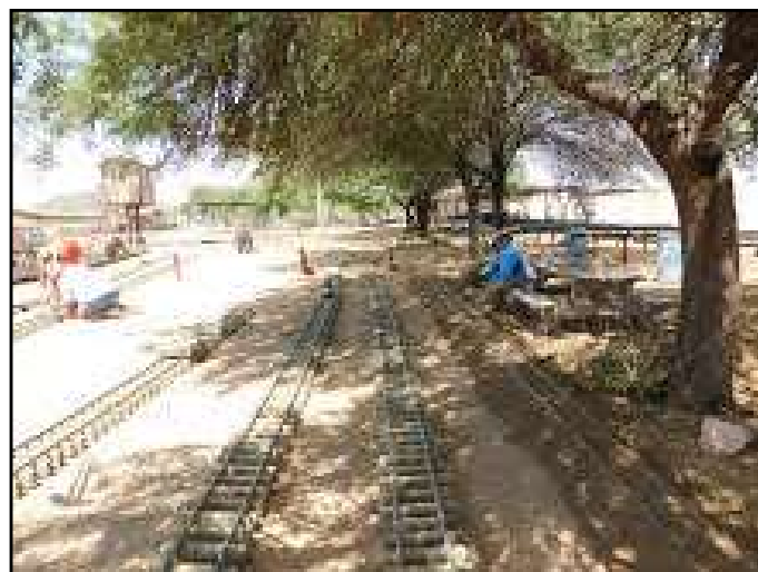
More yard spurs have been installed up to the trees by the steam-up bays.
