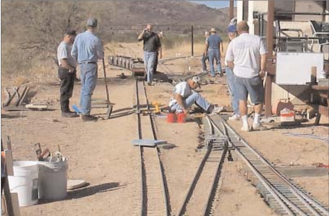
Bill Lowe and his merry gang of gandy dancers are seen replacing worn-out switches at Adobe Tower. More photos on page 3.
